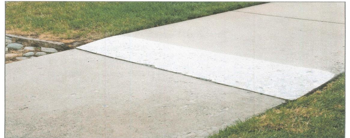
After Precision Concrete Cutting has completely and smoothly removed the trip hazard.
