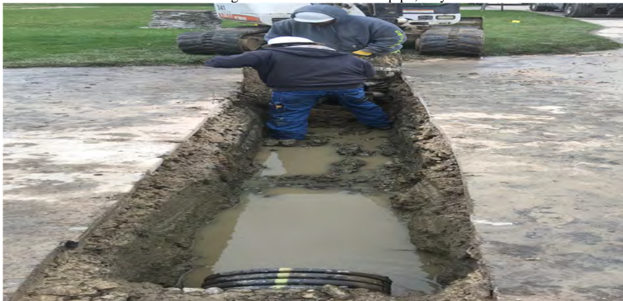
Location of broken storm pipe in front of 688 Wright Street
