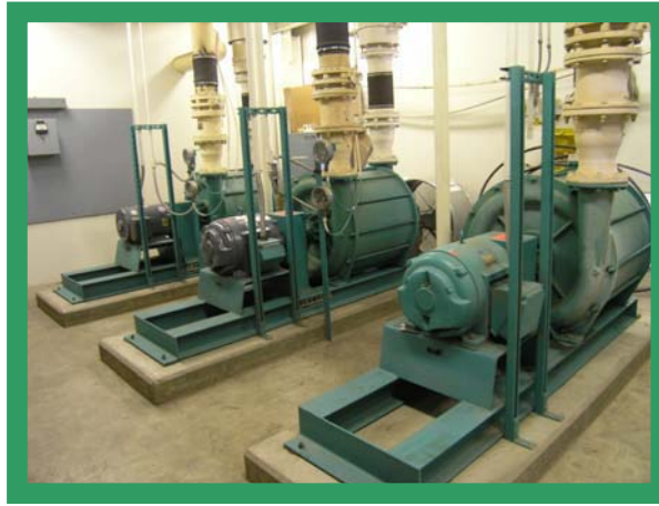
Energy Figure 13. These blowers are the main source of energy consumption at the sewer plant Source: Tim Burgener
